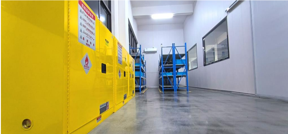
Low temperature battery storage
